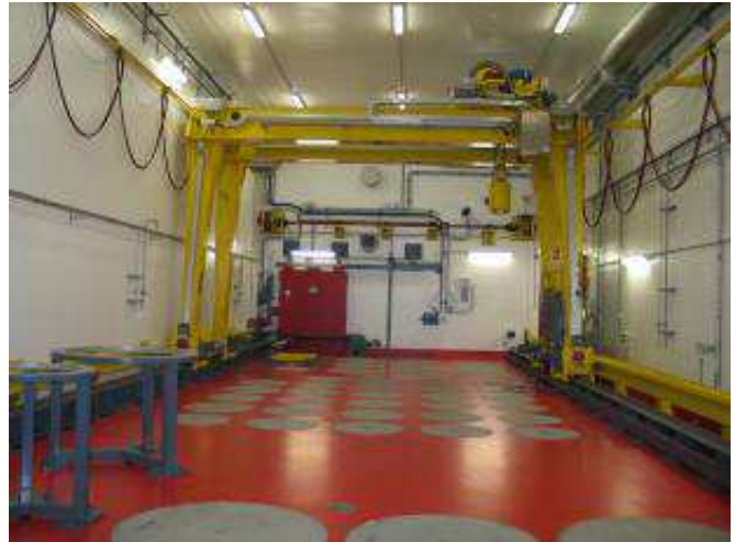
Figure 1.6 Heat producing waste storage
