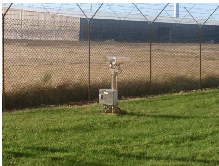
Figure 6.2 Part of the gas detection system
