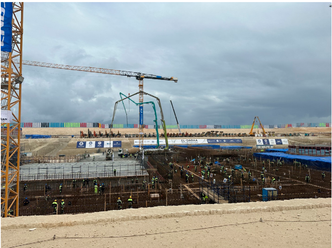
Pouring the first concrete into the foundation slab of Unit 4 of the El Dabaa NPP on January 23, 2024. Source: ASE
